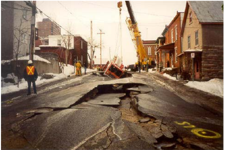
Damage caused by the release of pressurized water, from a corroded water main. Note the fire truck that came to the rescue.
