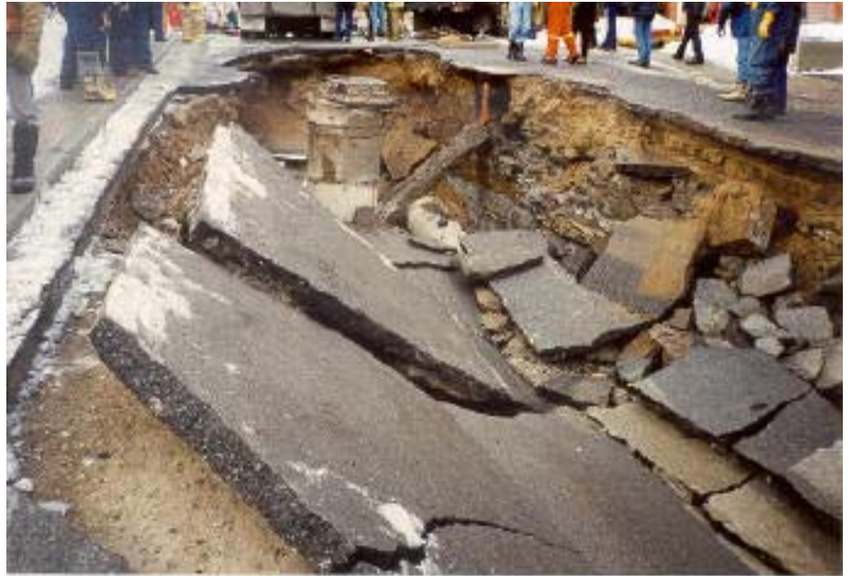
A closer look after fire truck was removed.
